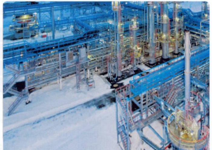
Hydrocarbon treatment facility at a Lukoil refinery in Siberia
